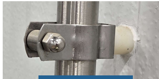
Minerallac clamp bolted to IMP wall with spacers
